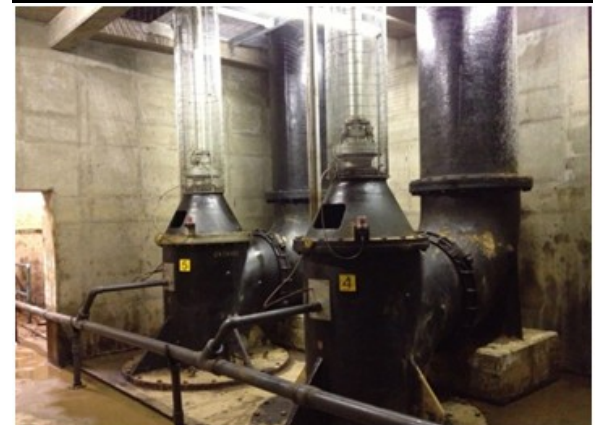
Original pumps from Allen Gwynnes
