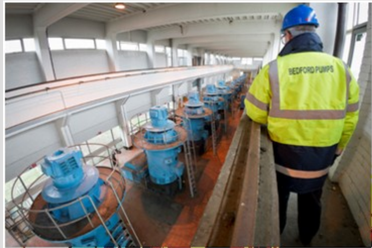
Crossness Intake Pumping Station before upgrade
