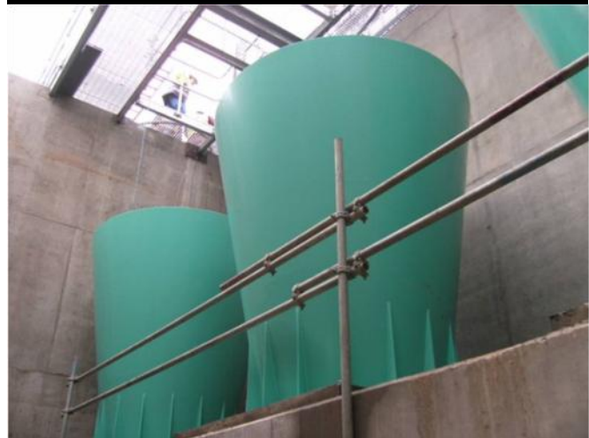
Canisters in place
