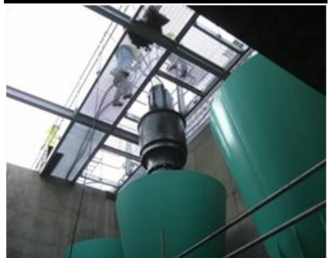
Pump into the canister at Minworth STW
