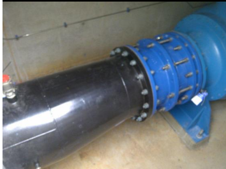
Pump installed in Brisbane, Australia
