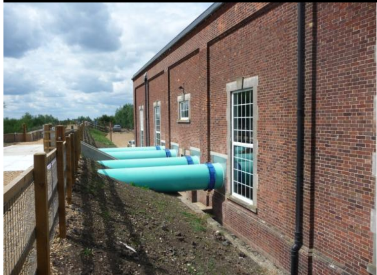
Discharge pipework at Welches Dam
