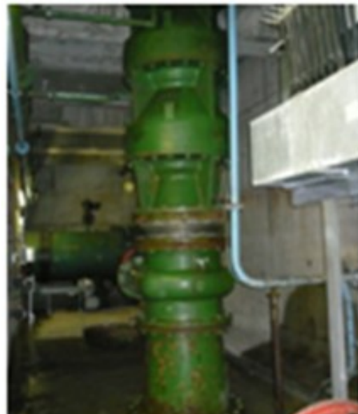
Fig 1. Existing pumps at Coppermills AWTW
