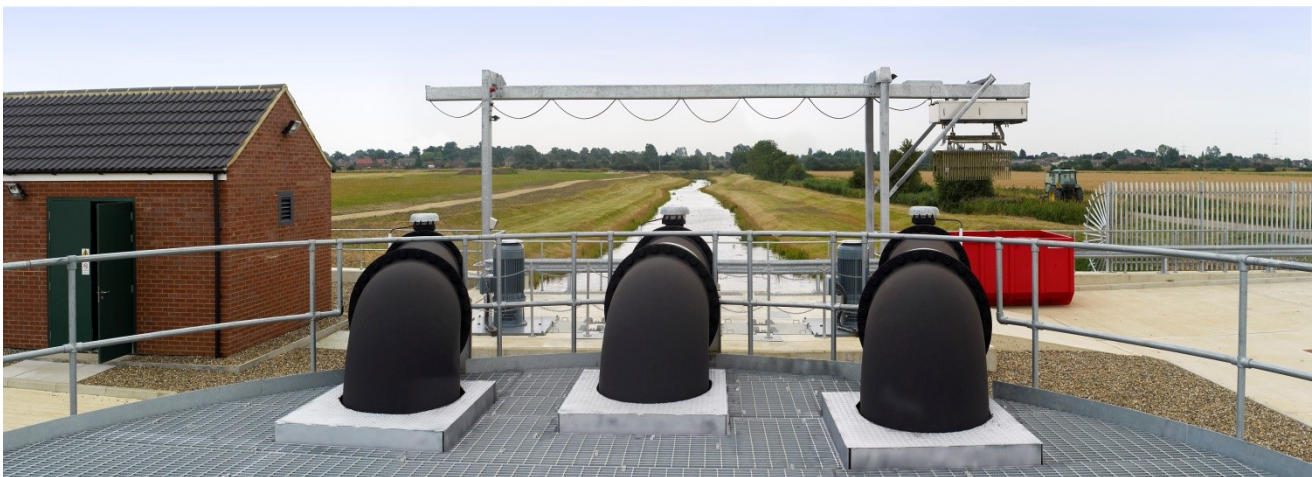
Fig 1. Puny Drain Pumping Station
